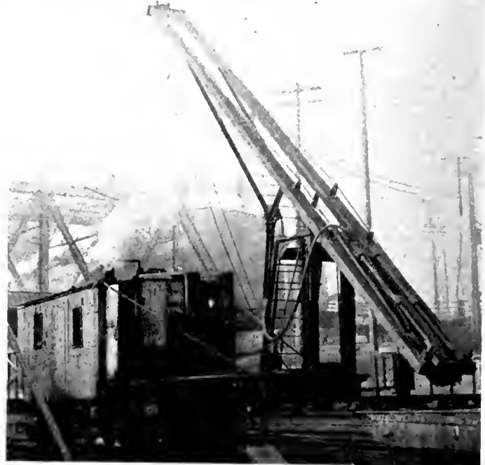
Leads are hinged to facilitate transportation. Folding is accomplished by movement of the hammer within the leads.
